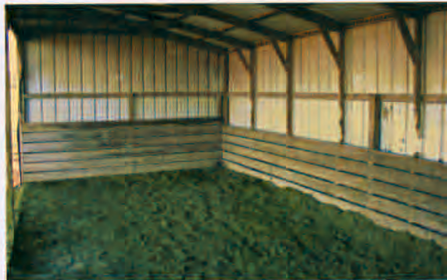
To keep horses from kicking through metal siding on a run-in shed, install kickboards at least four feet high inside the shed.
