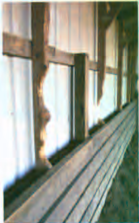
Chewed or rotten boards pose health hazards to horses and should be replaced immediately with hard or treated lumber.
