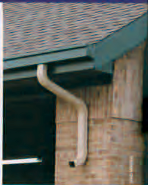
Gutters, overhangs, and sloping the landscape away from the run-in shed's entrance will keep the inside dry and safe for horses.
